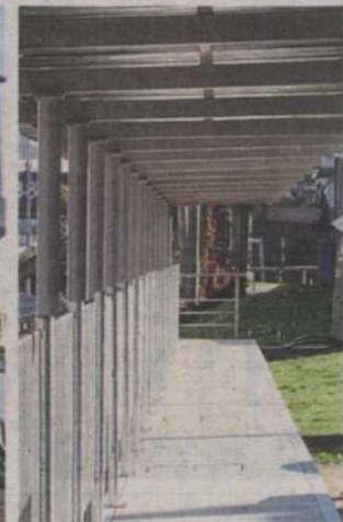
The covered walkway links the commercial areas of Bandar Puteri 1 and Bandar Puteri 4 in Puchong.
